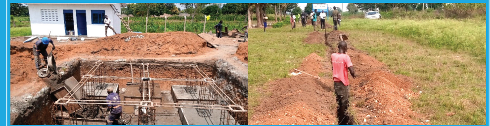
Fig 2: The Skilled and Unskilled working during construction of Adibo water Pump station
