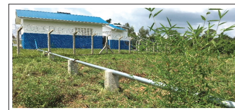
Fig 1: Adibo water source and Pump station
